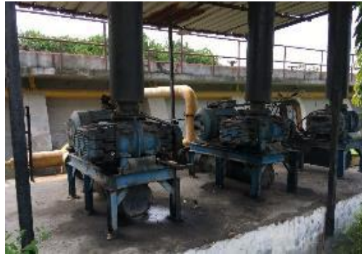
Blowers for Aeration Tank
