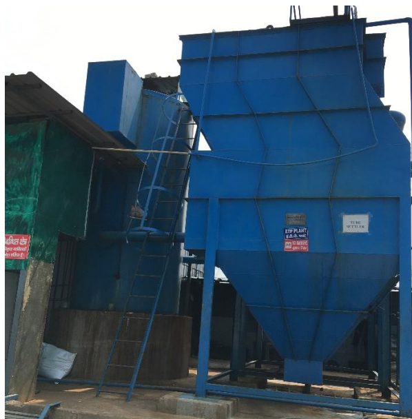
Flocculator and Tube Settler
