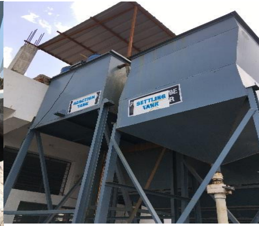
Reaction and Settling Tank
