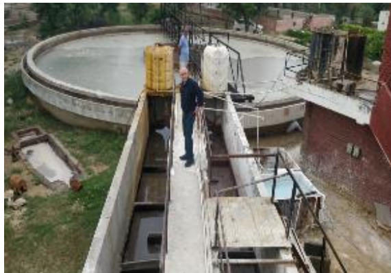
Flocculation Channel & Clarifier
