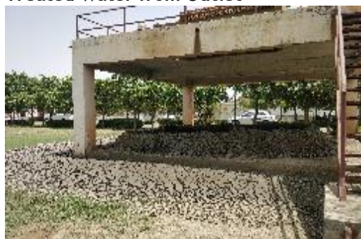
Sludge Dewatering using Filter-Press
