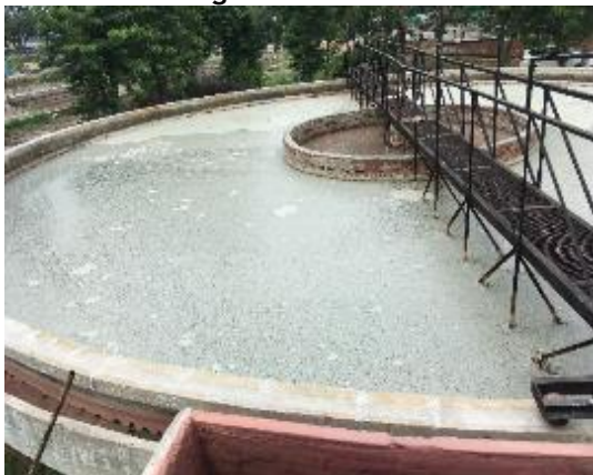
Final Sedimentation Tank (Secondary Clarifier)
