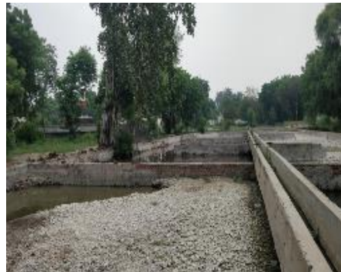
Sludge Drying Beds
