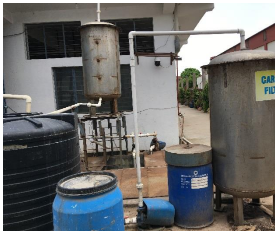
Sand Filter and Carbon Filter
