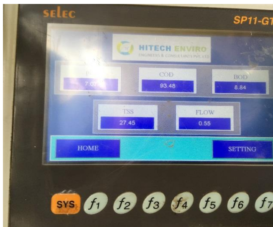
Online Monitoring Unit
