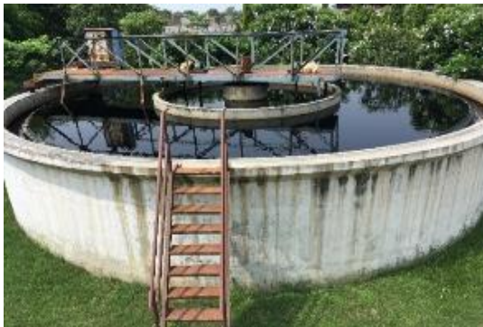
Final Sedimentation Tank
