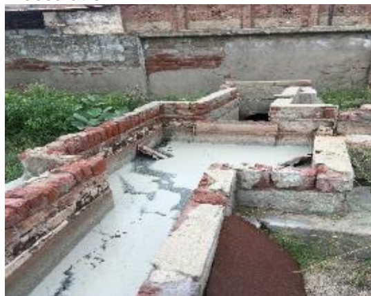
Outlet of CETP
