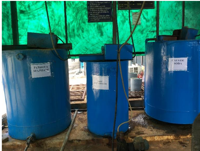
Chemicals for Flocculation
