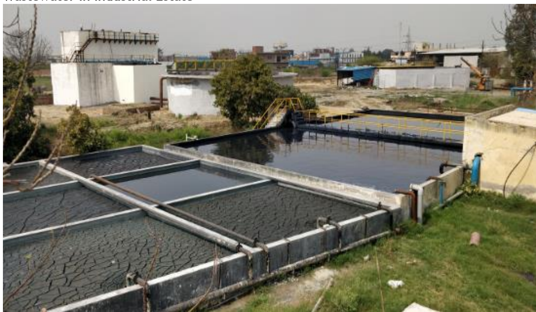
Sludge Drying Beds at CETP
