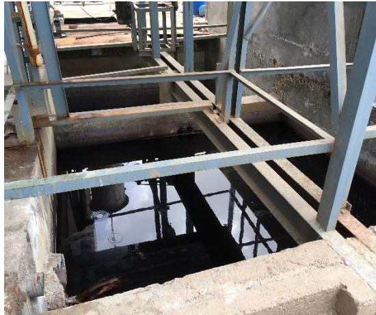
Equalization Tanks (sedimentation)
